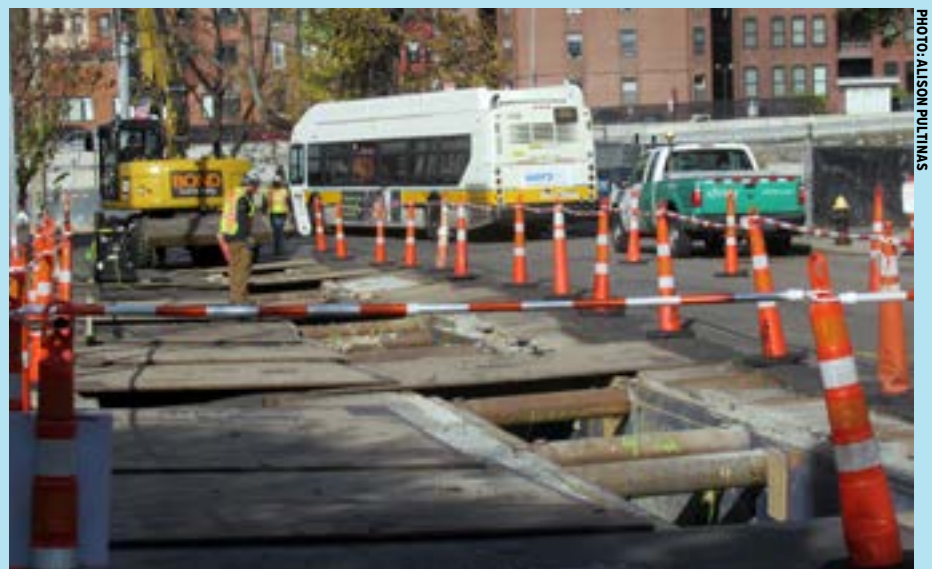
The #55 bus threads its way around an excavation trench on Ipswich Street.
