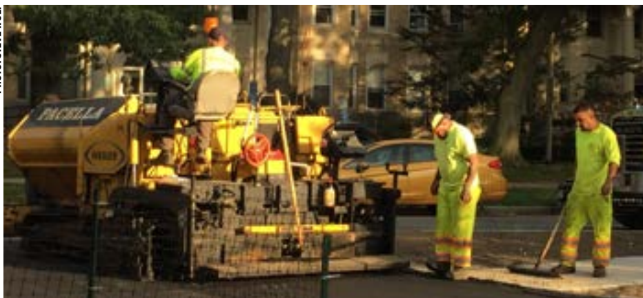
A crew put finishing touches on the repaving of Agassiz Road on October 11. Charter has since reseeded most of the roadside lawn strips, barren for years.
