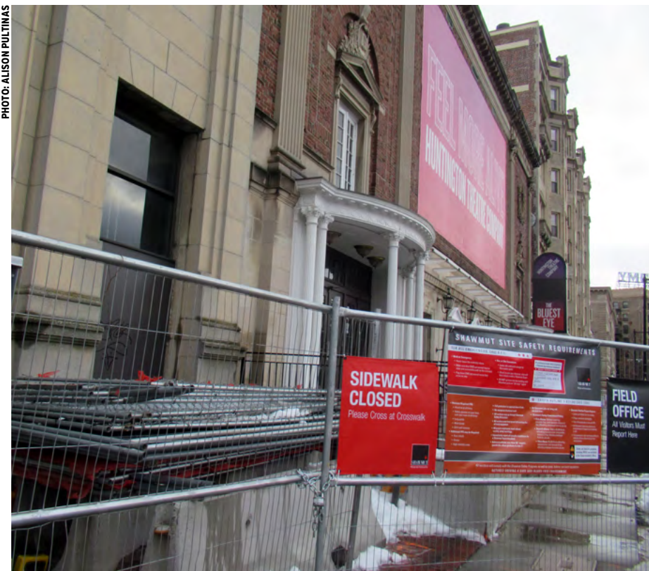
Renovation of the Huntington Theatre has closed the sidewalk on the south side of Huntington Ave. Plans include an addition to the theater's rear west wing, interior renovation, new roofs, and an enlarged front terrace. All fixed theater seating will be replaced, but other historic elements will be salvaged.
